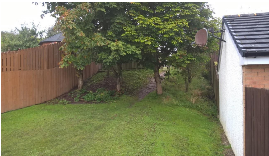
Figure 3 Steep slope to the top of the embankment
